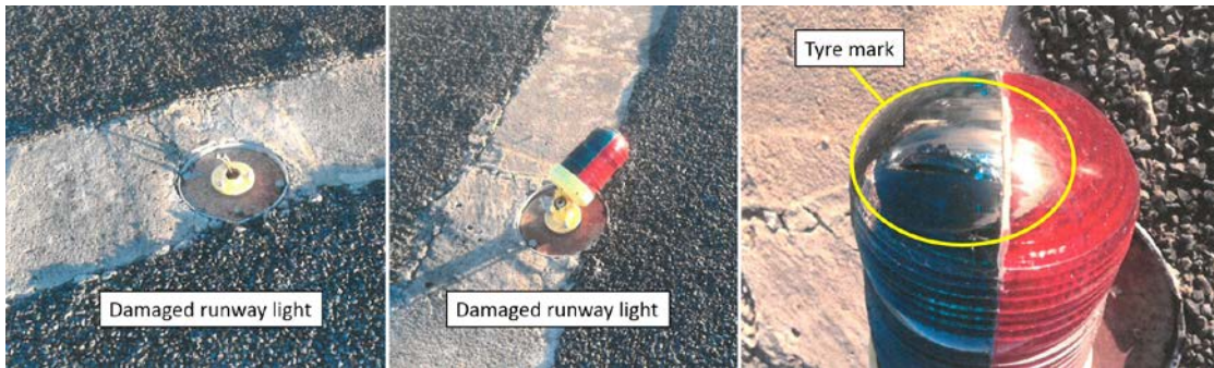
Images shows the damage to the runway threshold lights (left and centre), and a tyre mark on a damaged light (right). Source: Airport operator, annotated by ATSB
