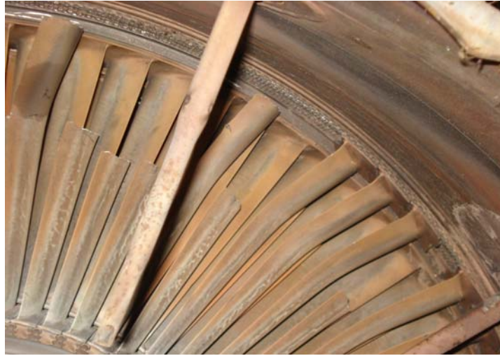
Photo 6: Turbine blade damage and some rubbing observed during the teardown inspection.
